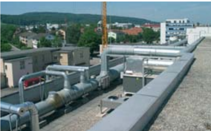
Exhaust air channels in Dübendorf (Switzerland)
