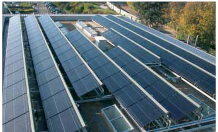
Solar captors on the roof of the lower part of the building.
